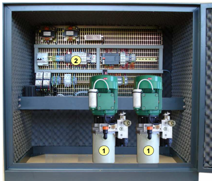
1- Special hydraulic group, 2- Control panel with AT224 PLC, 1 access, 2 bollards (example)
